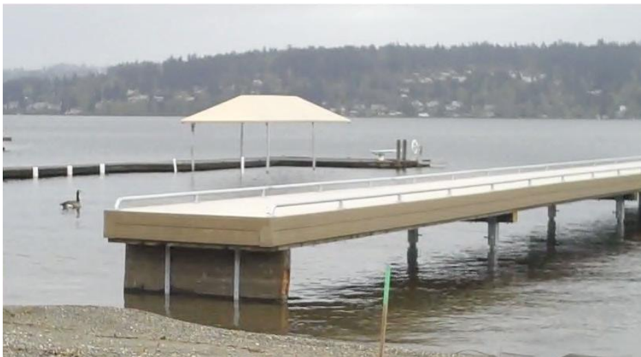
Figure 2 - Dangerously Exposed Dock
