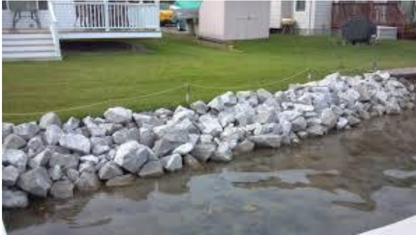
Figure 3 - Shoreline Stabilized by Angled Rip Rap
