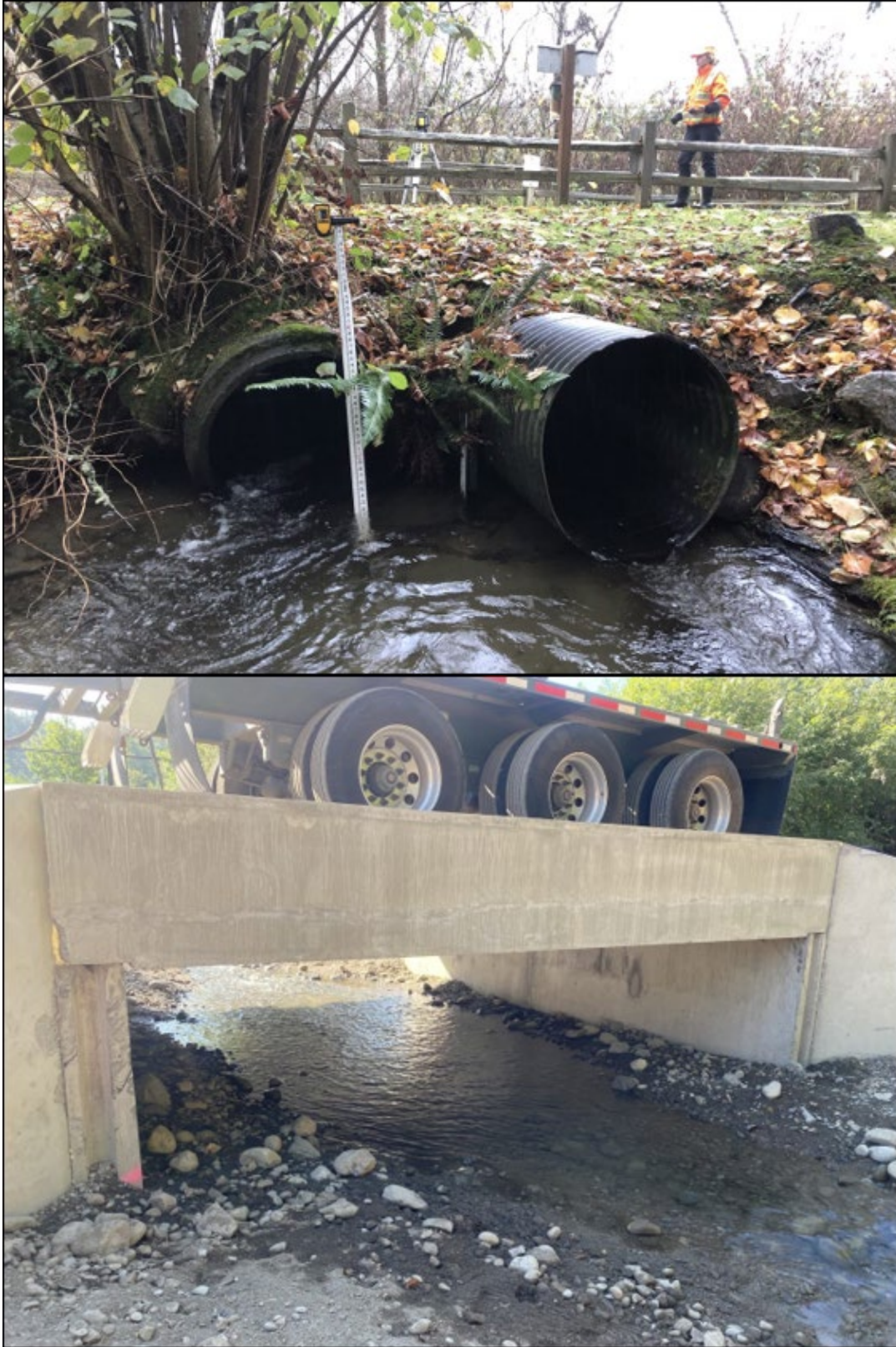
Before (top) and after (bottom): Culvert replacement with fish-friendly box culvert on Ebright Creek under East Lake Sammamish Trail, 2022
