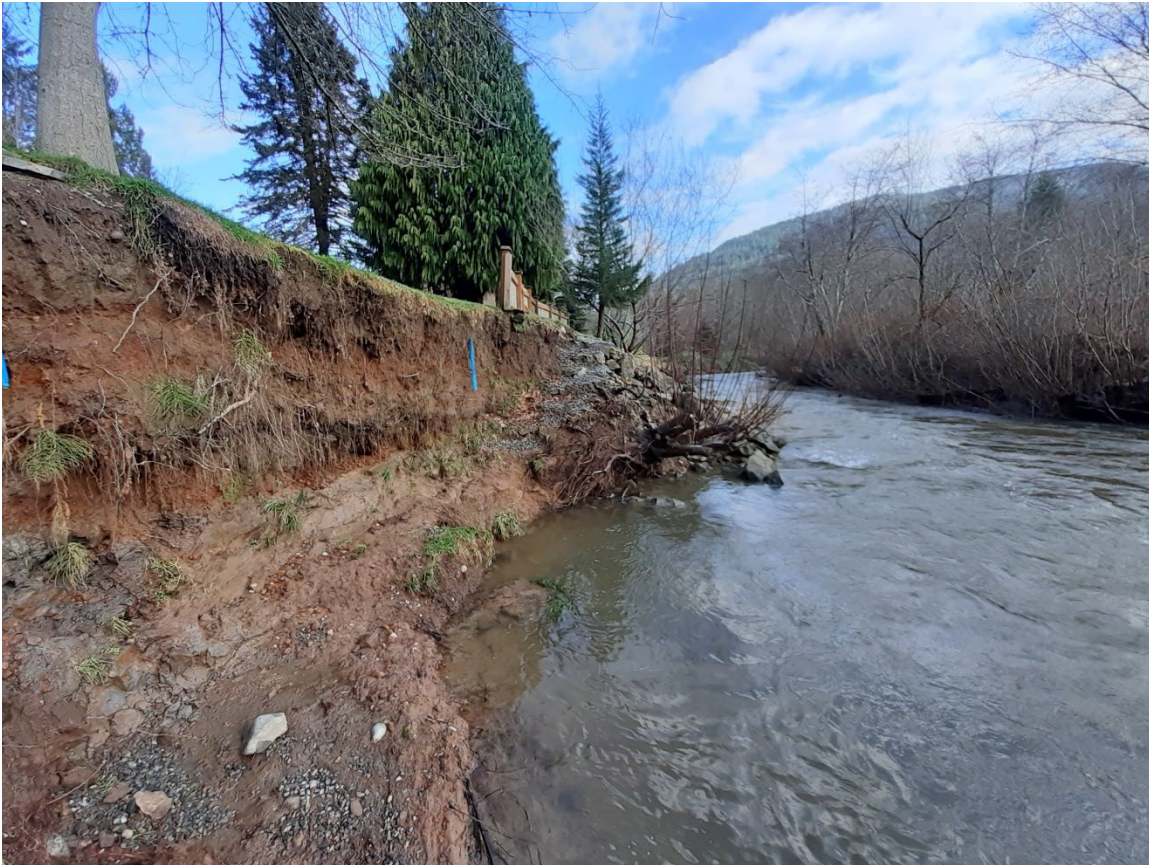
Erosion from Issaquah Creek flooding, January 2021
